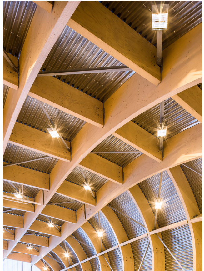
Figure 3. Multiple glued and curved Kerto members in roof structures of a sports hall.
